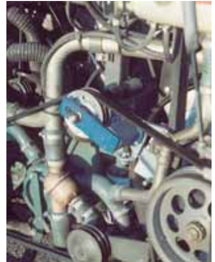
Belt tensioner on belt drive between diesel engine and AC-compressor
